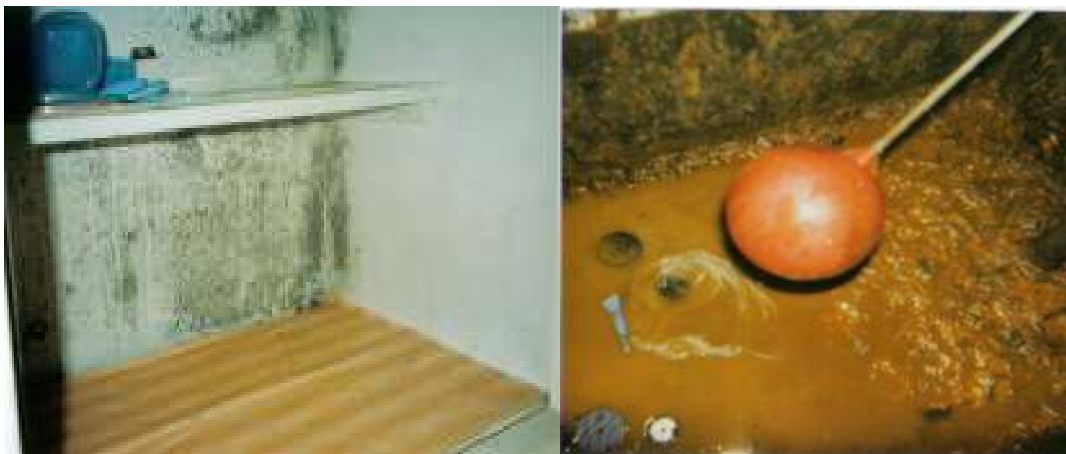
left: mould growth & dampness in clients' home; right: clients' cold water tank
